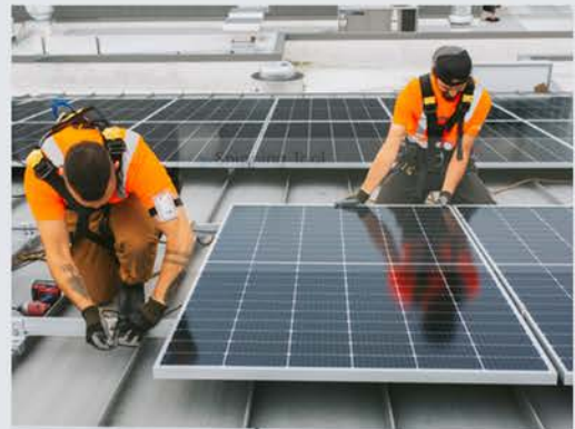
Solar installation at BLI.
