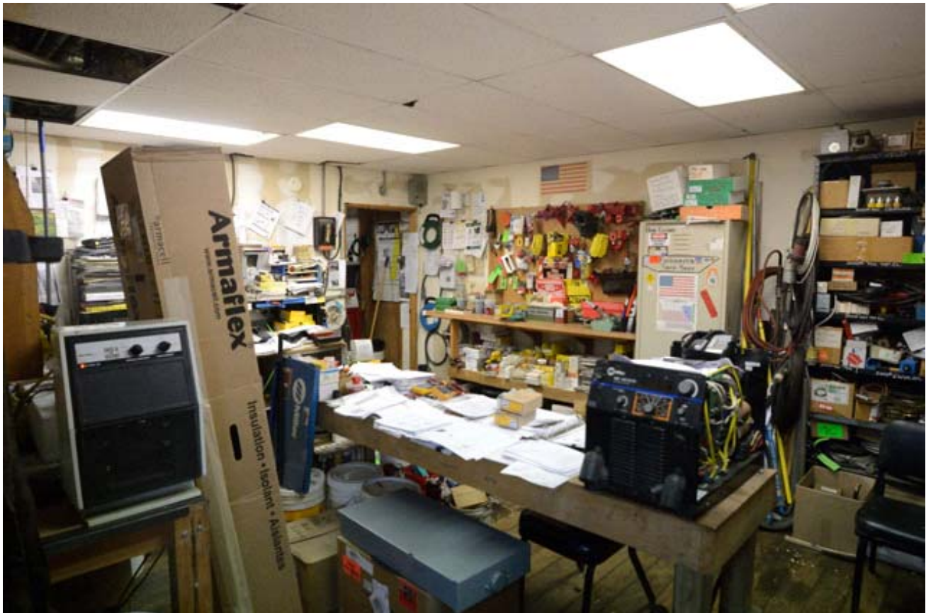
41. First Floor, Electrical Shop, View Southwest
